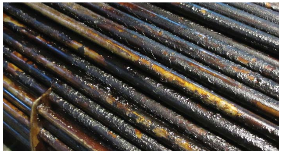
An oil cooler covered by sludge from oil-aging products
