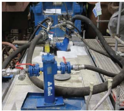
Bypasses on a turbine bearing of a large steam turbine
