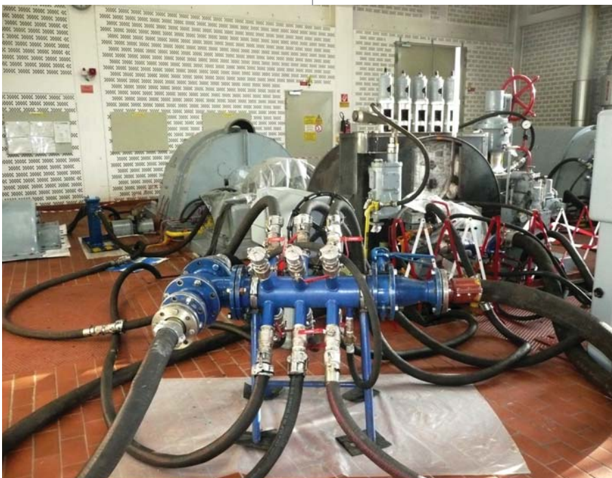
Manifolds and temporary connections on a small steam turbine
