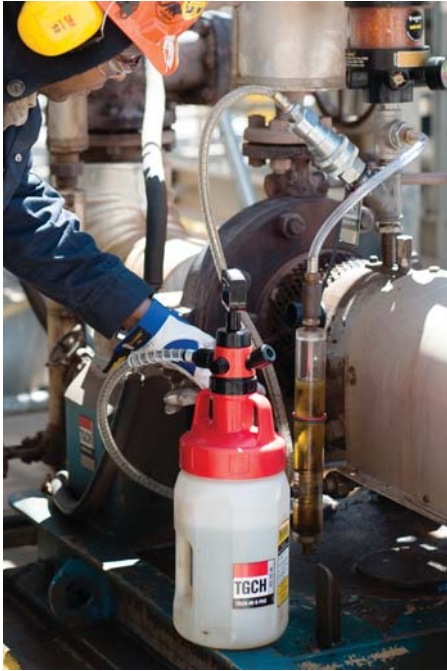
Sealable and refillable containers are now the plant standard for all oil top-ups.
