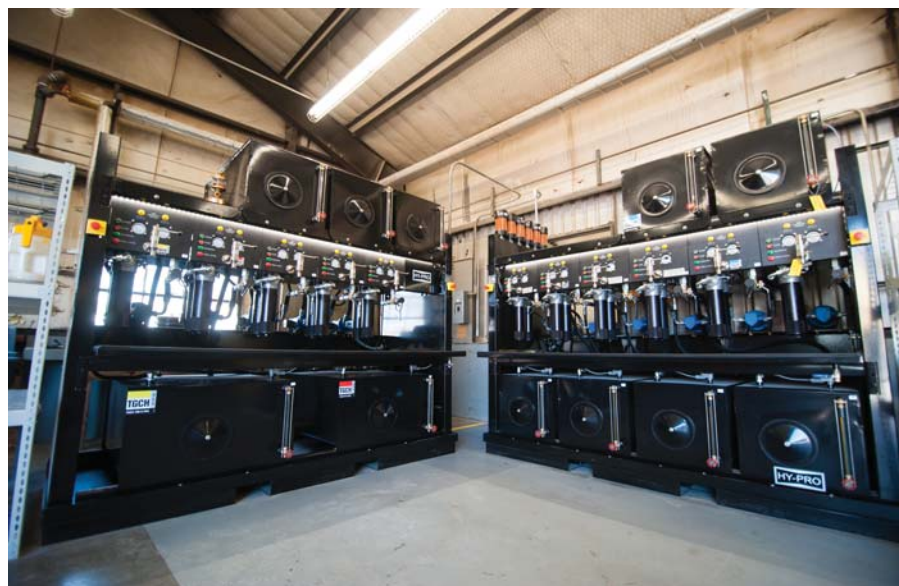
The renovated lube room offers better lubricant storage.
