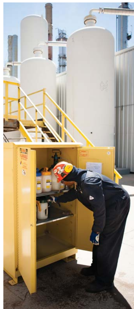
This new satellite storage cabinet is designed for storage of small oil containers and grease devices.
