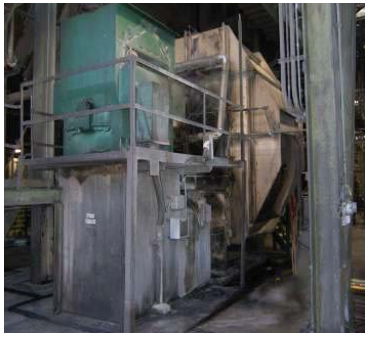
FIGURE 8. A large centrifugal fan
