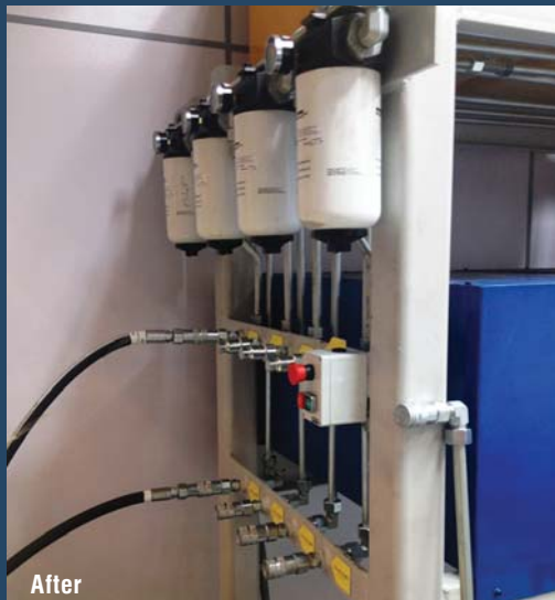
An absolute filtration system was designed to improve the oil cleanliness level.
