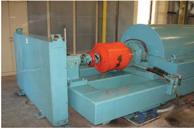
The planetary gearbox assembly with the guard shroud removed for viewing
