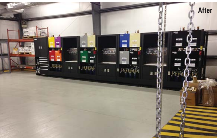
IKEC's new lube room features a filtration system with 16 filtering compartments, tanks and dispensers.
