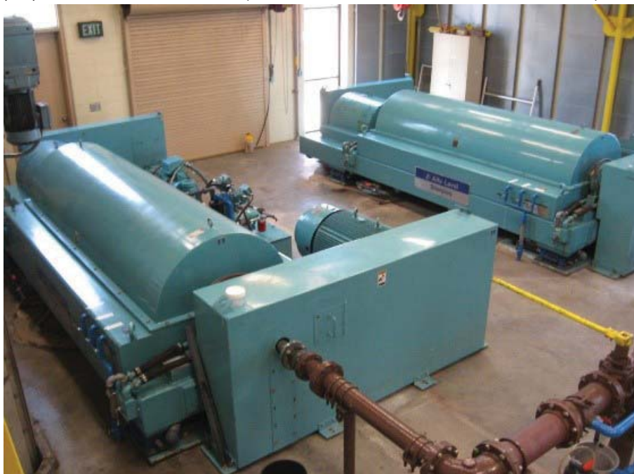
Sludge dewatering centrifuges
