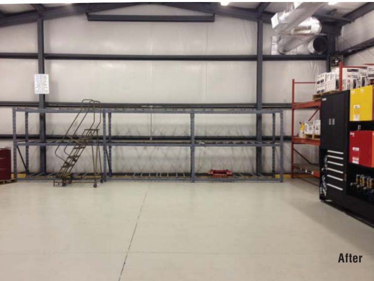
Among the modifications IKEC made to its lube room included a new floor coating and first-in/first-out drum storage racks.
