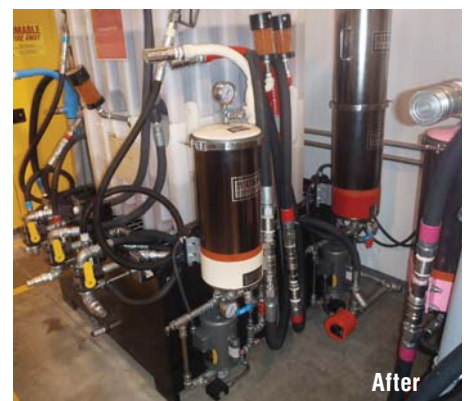
Dedicated storage tanks with filtration capabilities are now in use.
