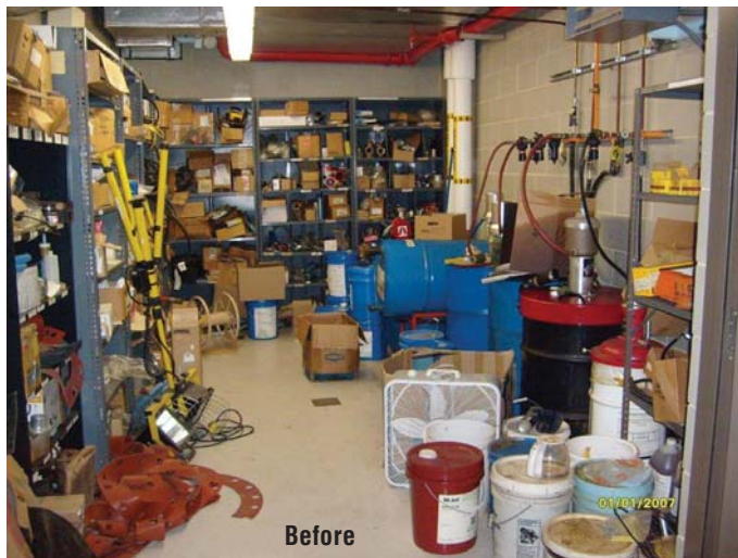
Before UOSA's lube room was revamped, its oil storage was an unorganized mess. The new lube room is more user-friendly and allows lubricant inventories to be better controlled.
