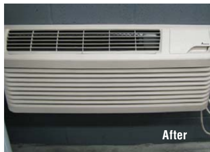
The mill's lube room is equipped with an HVAC unit, which provides positive pressure, a constant temperature range and low humidity.
