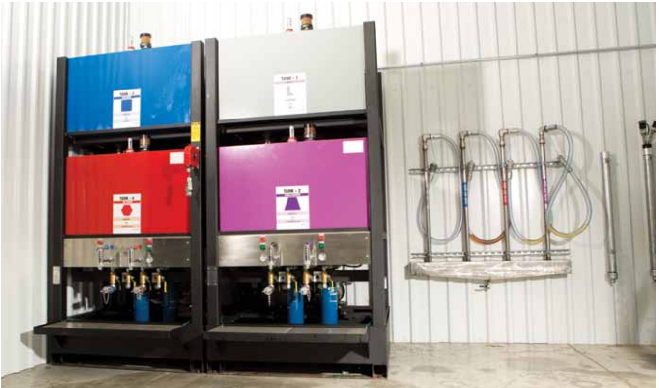
The non-food-grade oil storage units are complete with desiccant breathers, level indicators, pumps and filters for each container. There are no connections between tanks for cross-contamination.
