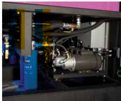
Pumps and filters are below each storage tank. Every tank has its own pump and filter.
