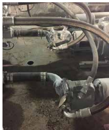
Hoses should be installed at the pump outlet prior to entering the manifold or main header.
