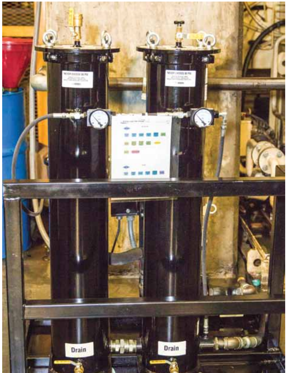
A kidney-loop system was installed to make it easier and more cost efficient to manage and maintain filters.
