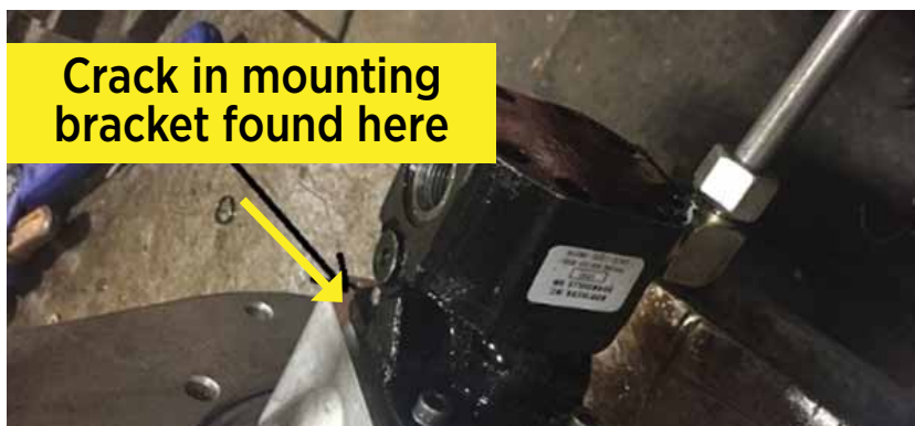
A pump with a cracked mounting bracket led to shaft misalignment and a worn seal.
