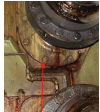
Figure 5. An example of leaking gearbox seals
