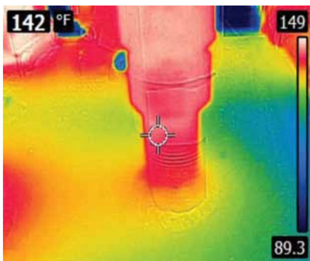
Figure 5. Image showing the tank line temperature of a check valve
