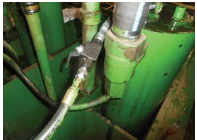
Installing a manual valve in the line to a prepress ram helped troubleshoot a pressure problem at a plywood plant.
