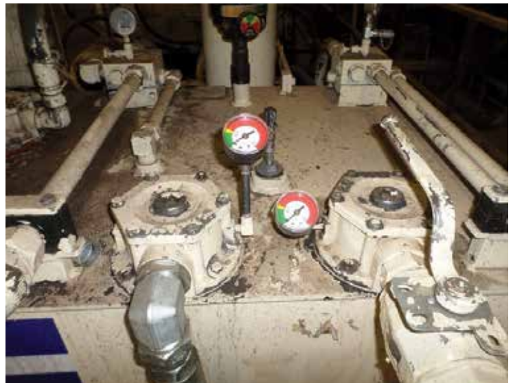
When gathering information, be sure to check the condition of the filters.
