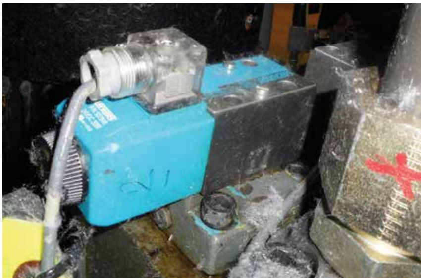
A blown fuse on a solenoid-operated valve resulted in unnecessary downtime at a plant in Arkansas.
