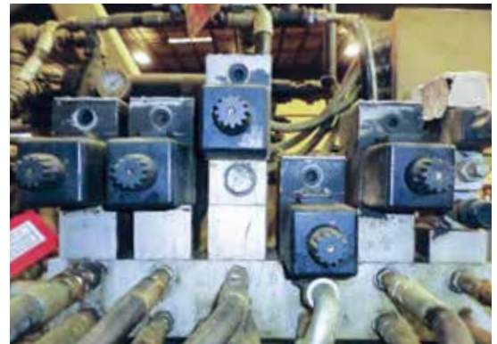
Valves located in a stack may look alike but perform completely different functions.
