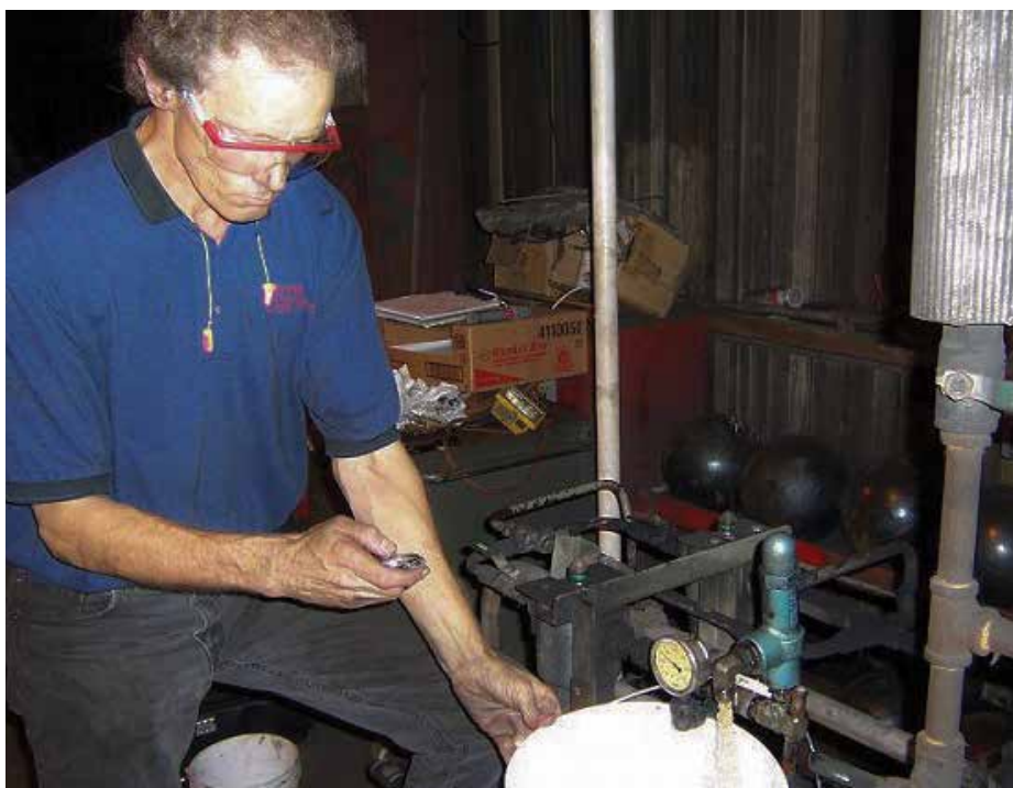
Check the oil flow out of the relief valve's tank line to assess whether a fixed-displacement pump is worn.
