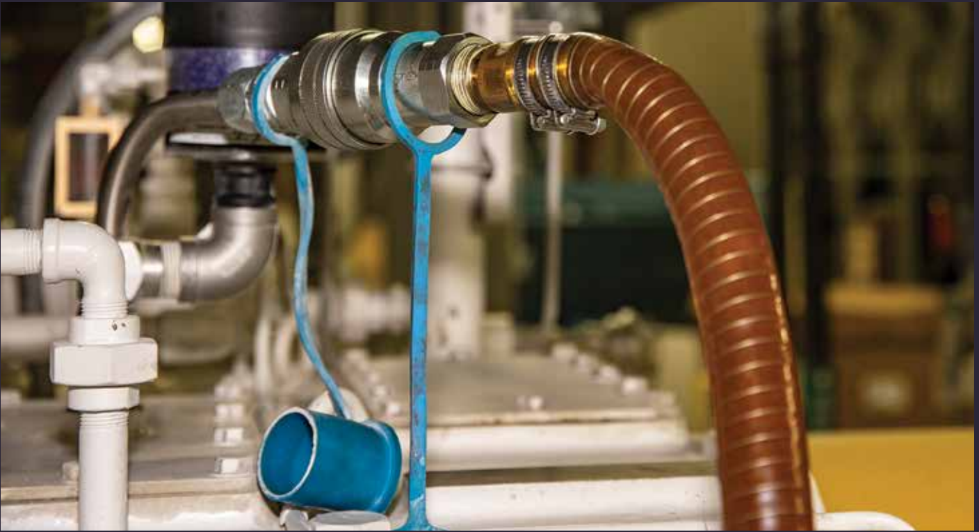
The filter cart connection on one of the breather mounts
