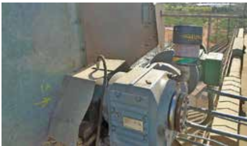
Figure 6. An exposed gearbox with a desiccant breather installed
