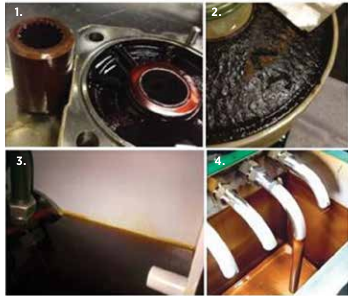
Varnish deposits on hydraulic pump (1), filter element (2) and tank walls (3 & 4)
