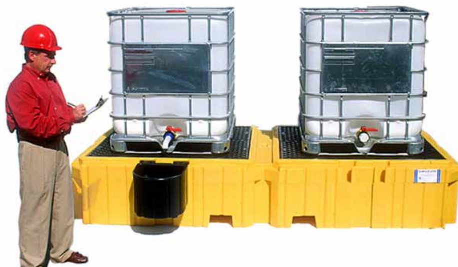
IBC in the plant.
