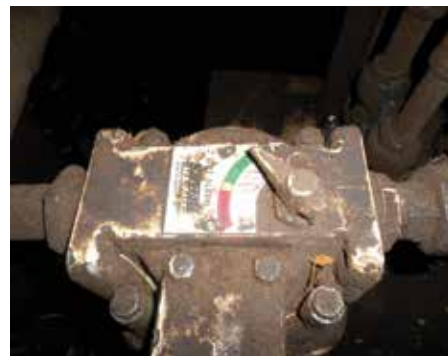
Visual indicators can fail and should not be relied upon.
