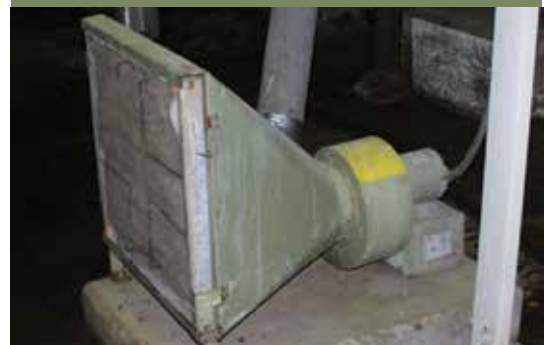
Tank-top vapor-extraction fan and panel filter.
