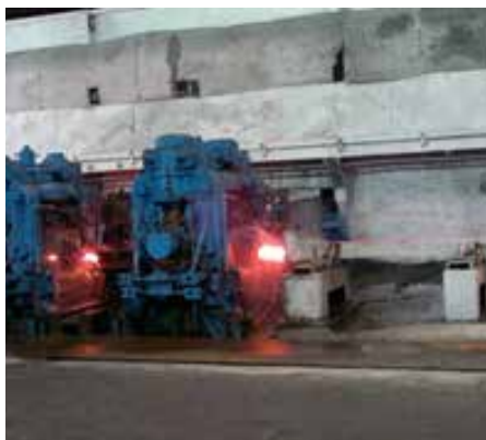
High pressure water exposure of bearing in the Mill
