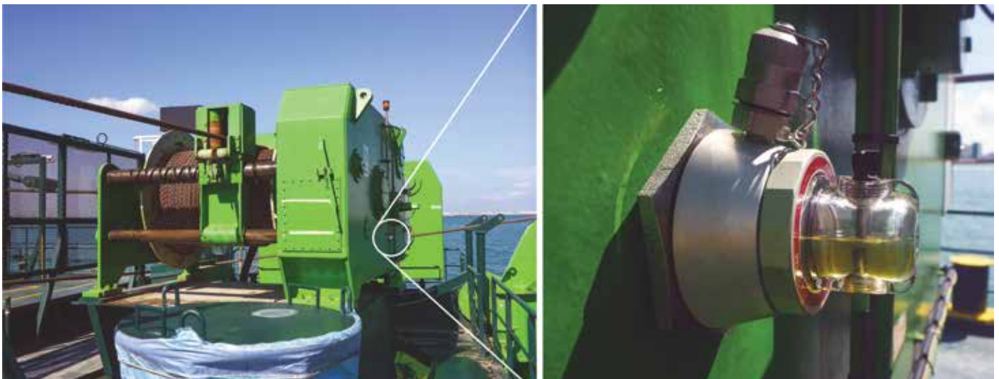
Figure 2 – One of the twenty-two winches with Luneta's Condition Monitoring Pod (CMP) installed.
