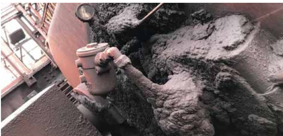
Figure 4. Large gearbox (4 reduction stages) used in a steel mill. Leakage around oil pump went unnoticed, ignored or just deferred for later repair. Little by little the gearbox drained of oil resulting in a thick dust cake. Oil pressure gauge was obstructed by the cake. Ref. Ronald van Druuten
