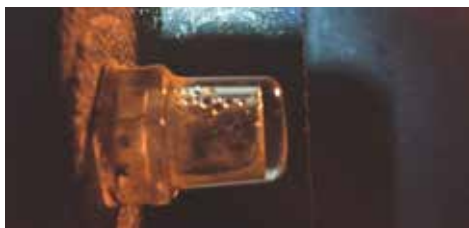
Figure 4. Keep oil levels tight. Allowing oil levels to drop will create more condensation as you can see from this picture.
