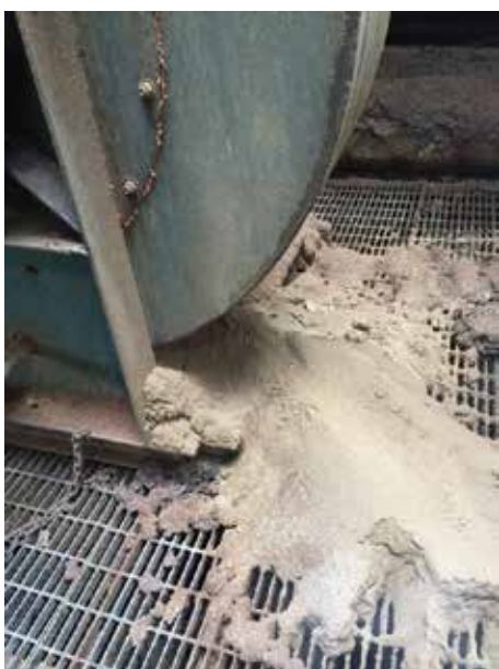
Figure 5. “Stop the domino affect” Repair, modify, or replace equipment before contaminants spread throughout the plant.
