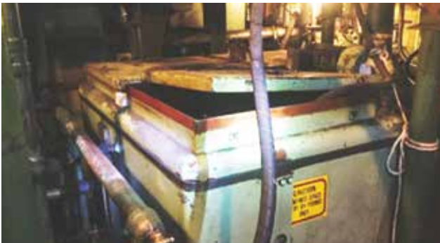
Figure 1. Temporary solutions can turn into catastrophic contamination. The picture shows the oil reservoir hatch opened with a hose running directly into the reservoir.
