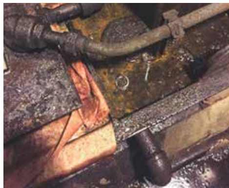
Figure 4. “Water will find a way” Keep standing water away from machine parts. Do not let a small water leak or containment drain problem destroy machine parts.
