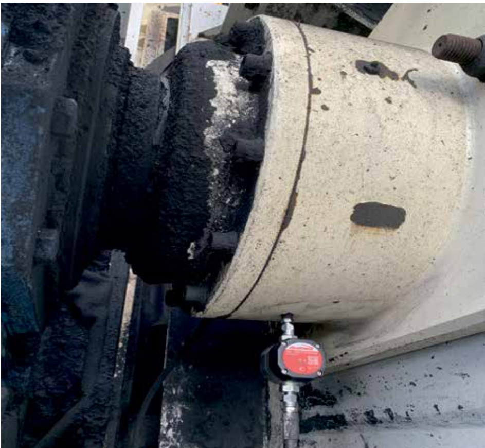
Endpoint on Apron Feeder. One major point of failure eradicated by a simple but powerful advance-warning system.
