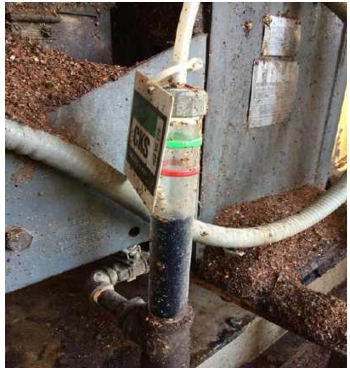
Can this level gauge see foam? Emulsified water? Oxidized oil? Correct oil level? Any concerns about the installation hardware? Ventilation? Sediment build-up between the elbow and the sump? Correct oil level?
