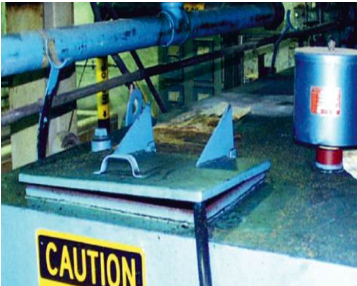
Photo of a hose obstruction
